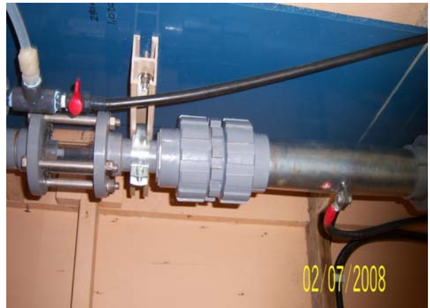
Holly Chlorine Generator
