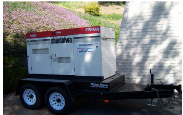
Pasadena Glen Reservoir Generator
