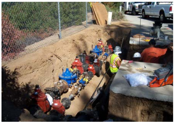
Ranch Top Road Interconnection Valves
