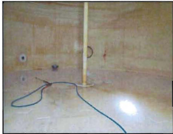
Interior - After Washout
